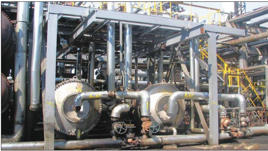
Figure 10 Two out of eight SHEs operating as visbreaking feed/bottoms interchangers
